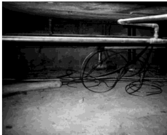
Figure 11-4—Excessive grounding conductor coil
